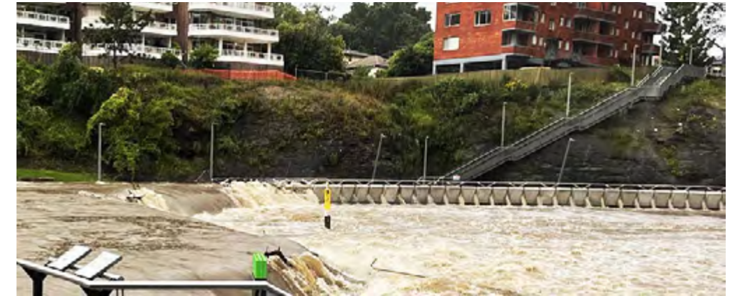
CHARLES STREET WEIR, PARRAMATTA Pathways are designed to withstand flood waters and fencing on top of the weir is designed to collapse under load to minimise upstream flood impacts
