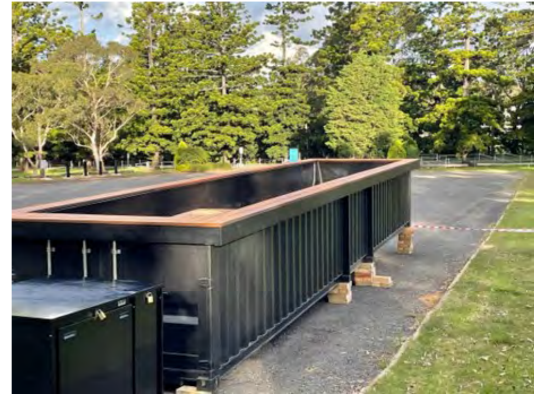
CONCEPT 4 First container and box housing filters and pumps installed on sloping site
