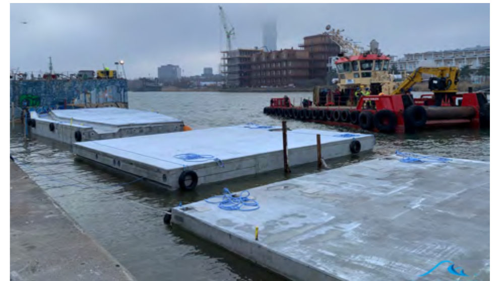
ALLAS SEA POOL, FINLAND The pontoons are floated into place within Helsinki Harbour
