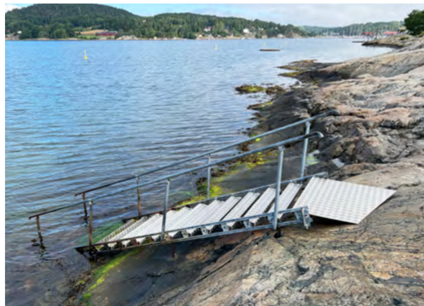
SON SPA, NORWAY A steel staircase enables safe access over the rocky foreshore into the fjord Image - Studio Octopi
